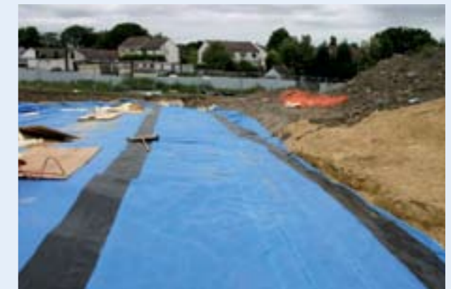
Stage 8: Protect the surface of the cell with sand and bury deep enough to prevent disruption in the future.
