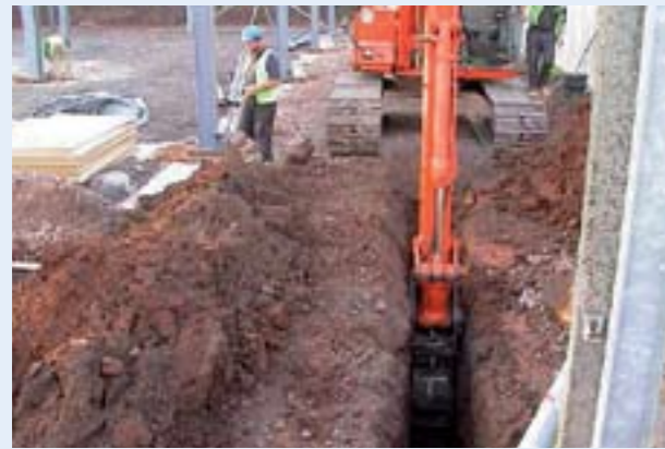
Stage 1: Excavate a trench, making sure that all the knotweed is contained.
