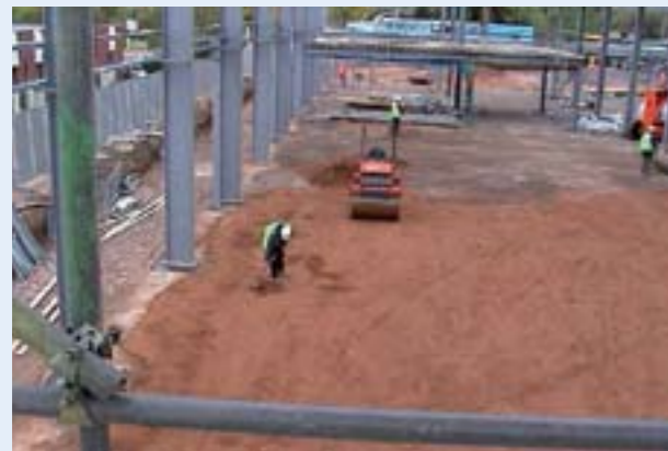
Stage 1: Protect the integrity of the root barrier membrane and prevent damage from 'heave' with a layer of sand.
