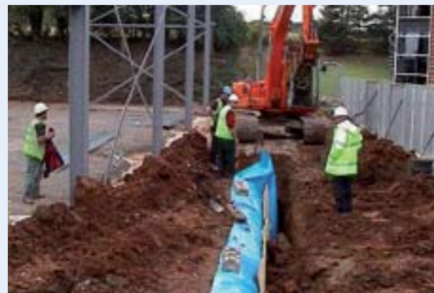
Stage 3: Support the root barrier membrane with shutter ply and backfill the trench.
