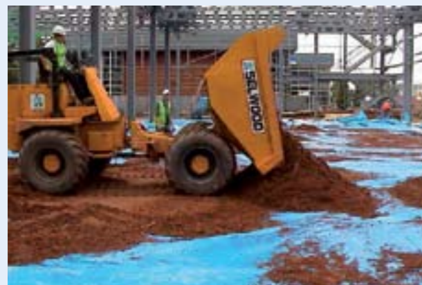
Stage 3: Apply another layer of sand over the surface of the root barrier membrane.
