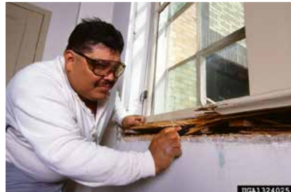
Figure 6.13.5 Termite damage to a window sill. The nest was located two floors below in the soil. Much of the wood had been consumed before they were detected. © Scott Bauer, USDA Agricultural Research Service, Bugwood.org
